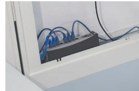
Router placed in systemscreen
