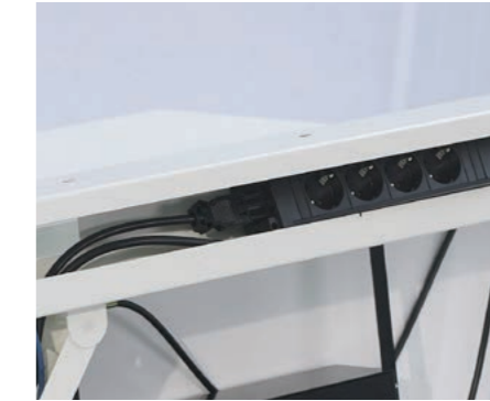
Cable gutter under work top
