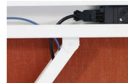
Cables from Elbow to under-work-top cable gutter
